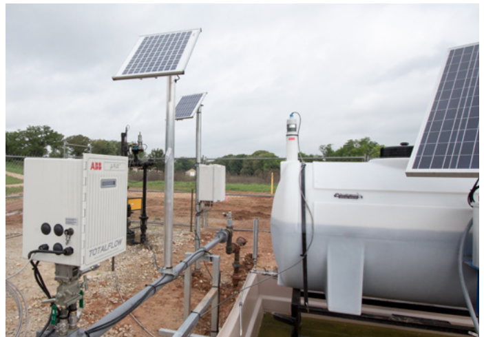
Fig. 1: Solar powered level application
