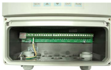
Figure 1 Terminal access on the LST400
